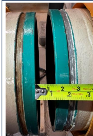
Figure 10 14-Inch Influent Plain End Pipe Separation at Grooved Coupling Location
