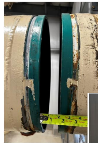
Figure 11 16-Inch Influent Plain End Pipe Separation at Grooved Coupling Location
