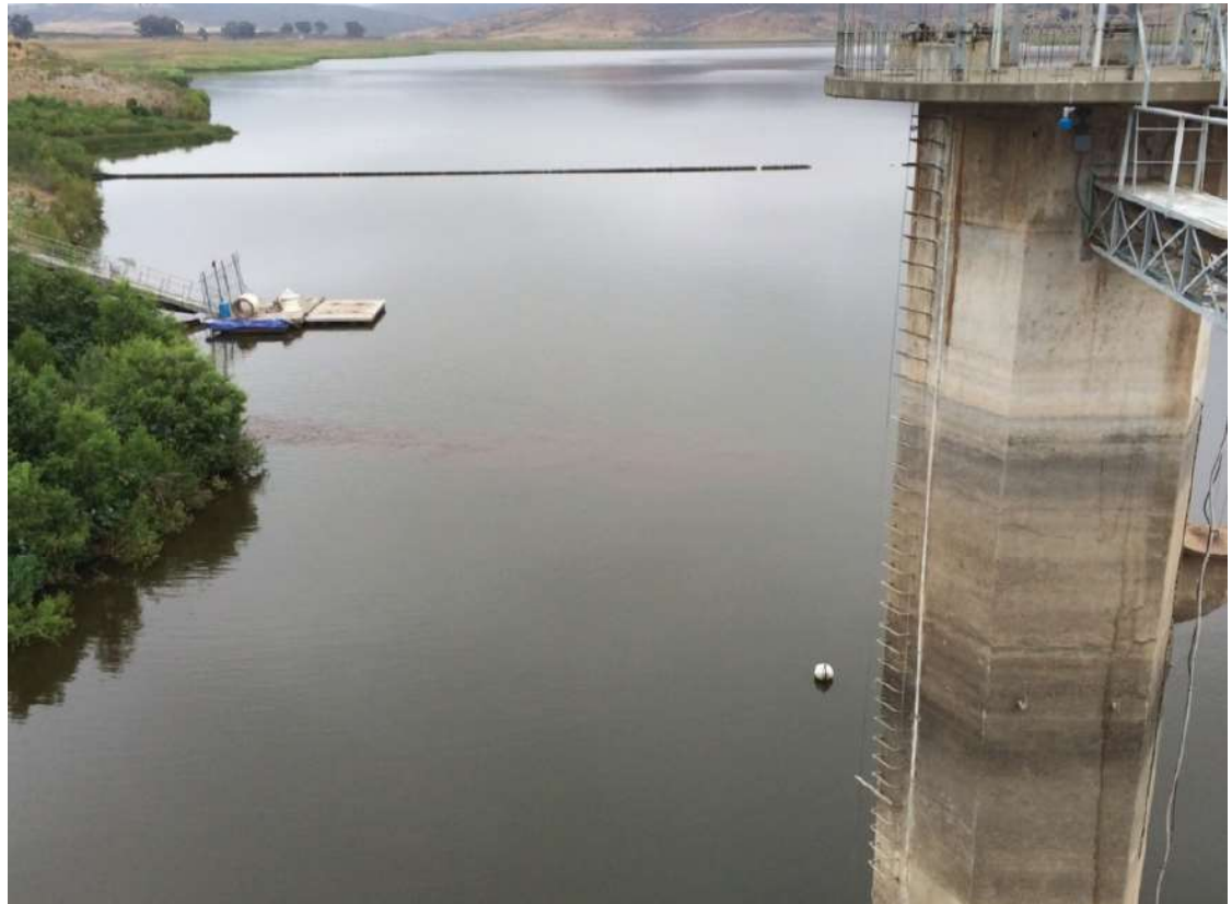
Figure 5.28 Filter Backwash Water Discharge Approaching Intake Tower
