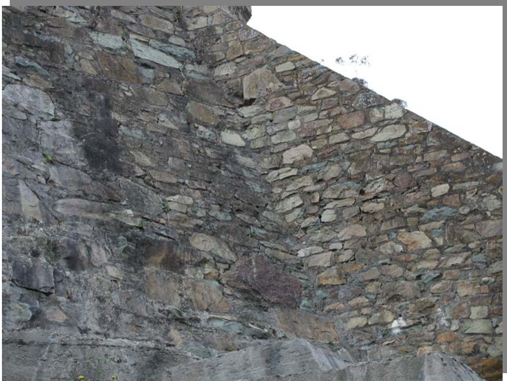
Photo 5 – Stone masonry on downstream side of dam, on right side of south spillway discharge channel (taken June 3, 2002).
