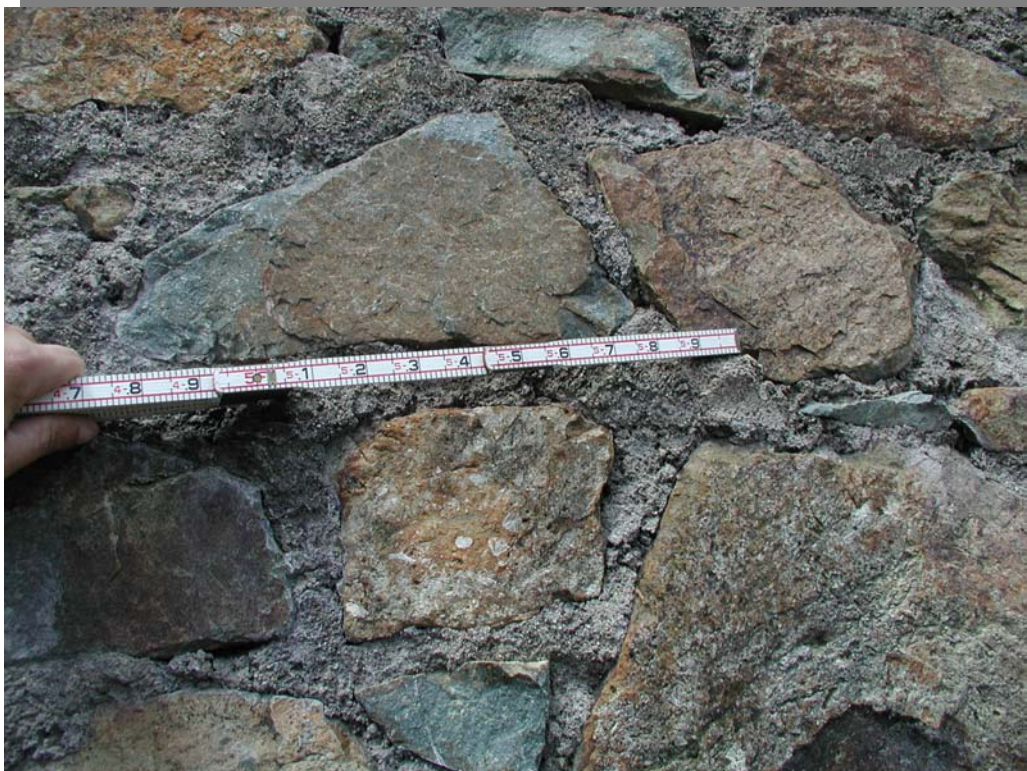
Photo 6 – Close-up of stone masonry shown in Photo 5, showing stones and mortar between stones (taken June 3, 2002).
